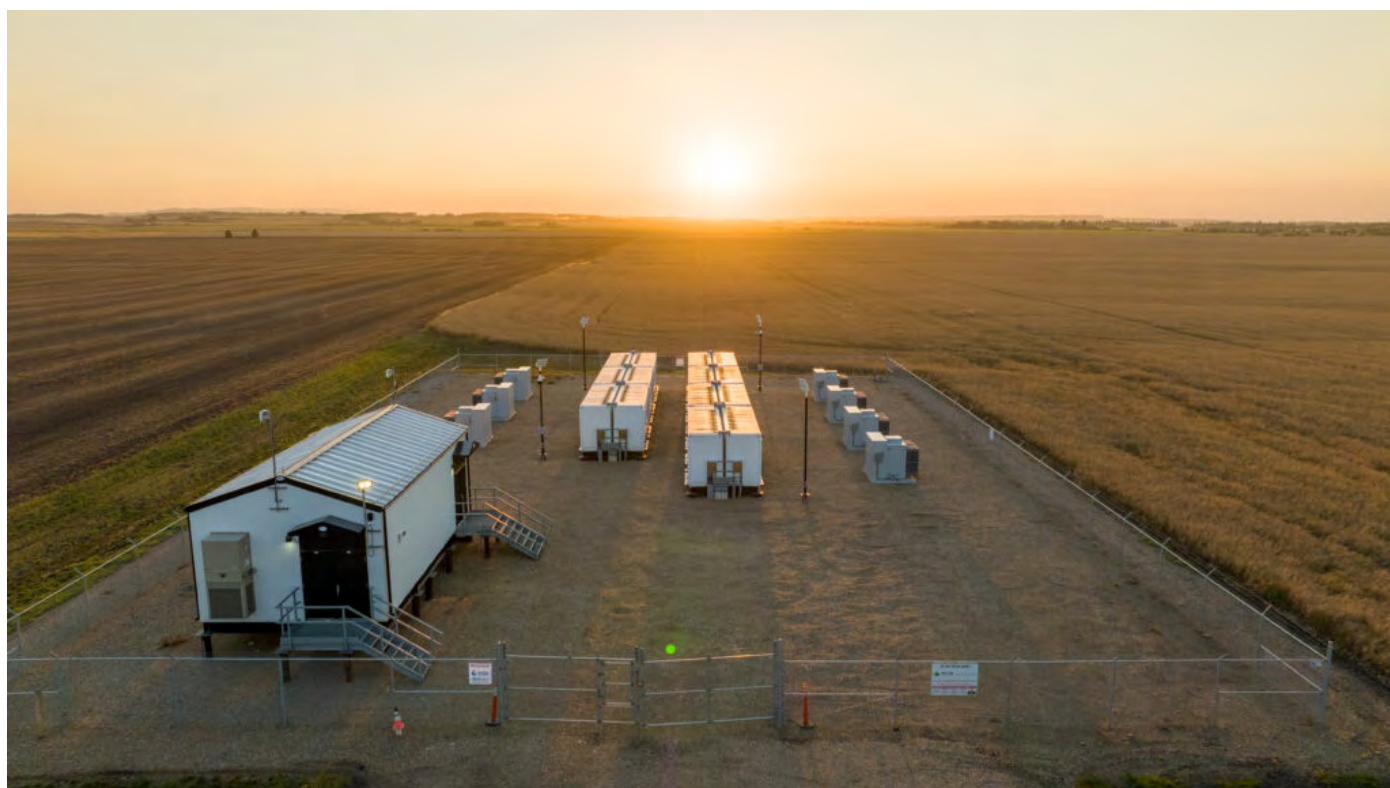
Enfinite eReserve Battery Storage Project (Alberta, Canada)
